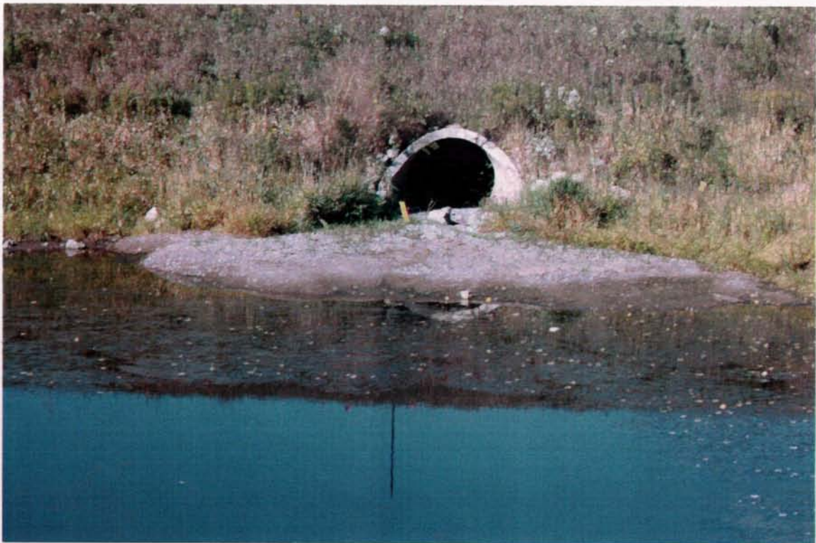
One of the Powers Lake storm sewer inlets on the east side.
