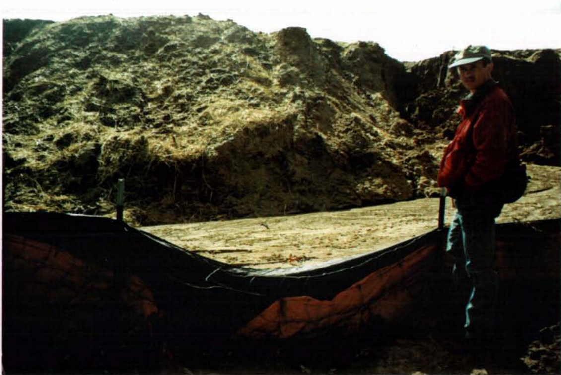
Figure 21. Erosion control at construction sites are essential especially in the lakeshed. [Top] Main inflow to Powers Lake heavily influences water quality. [Bottom] Photo was a 1998 construction project in the Powers lake lakeshed.
