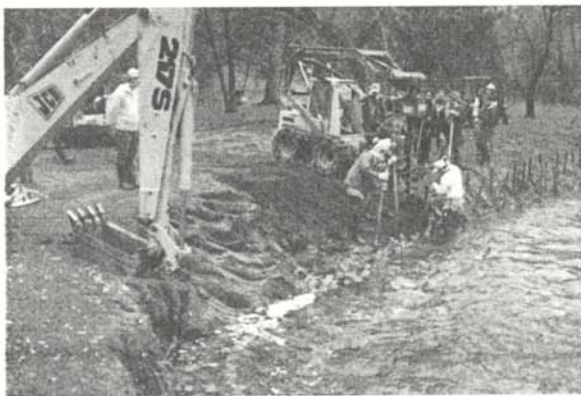
Reshaping the bank can be done by hand or with equipment. In this case, a backhoe is reshaping the streambank, followed by the placement of willow posts. An auger on the end of a bobcat drills holes for the willow posts.
