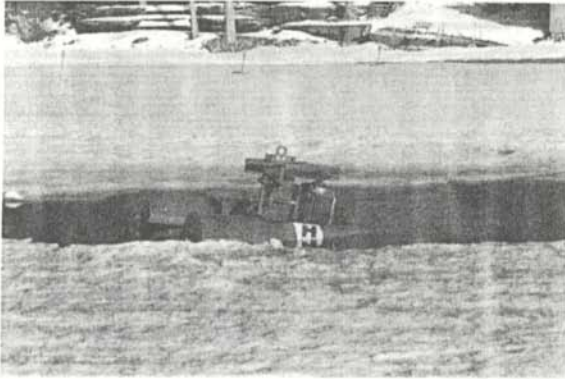
Another style of pump-and baffle-system uses an intake mounted on a floating platform. The hydraulic pump delivers low oxygenated lake water to the baffle component.
