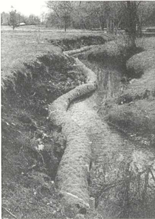
Coir fiber rolls can be used to stabilize the toe of a streambank. Bank reshaping and reseeding will complete the stabilization project. Coir fiber rolls are composed of loose coconut fiber from coconut husks, held together with coir fiber netting. In higher energy environments, rock is used. (From Don Knezick, Pinelands Nursery, Columbus, NJ. With permission.)
