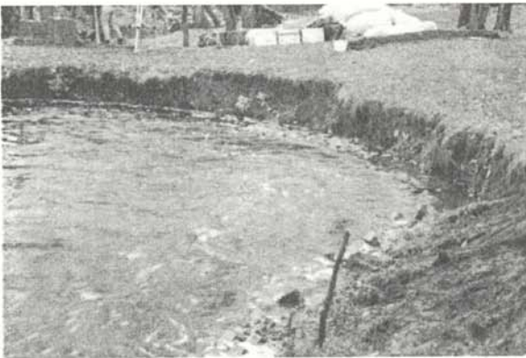
After toe protection is in place, the next step is to reshape the unstable bank.
