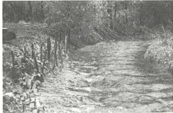
Willow posts and willow stakes are used to help stabilize streambanks. Their root systems stabilize the soil. Willows are often acquired from river floodplain areas. They are left soaking in water until they are used. They should be cut and inserted into the ground as soon as possible.
