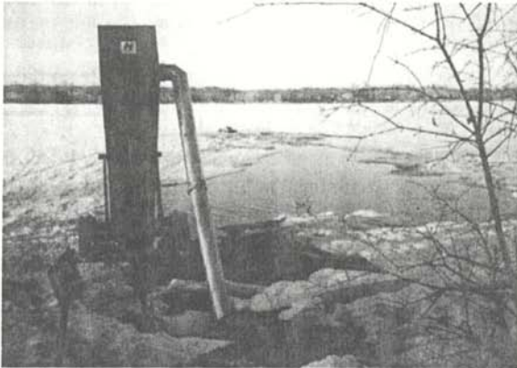
Lake water goes in at the top of the baffle and cascades back into the lake. (From City of Lakeville, Minnesota.)
