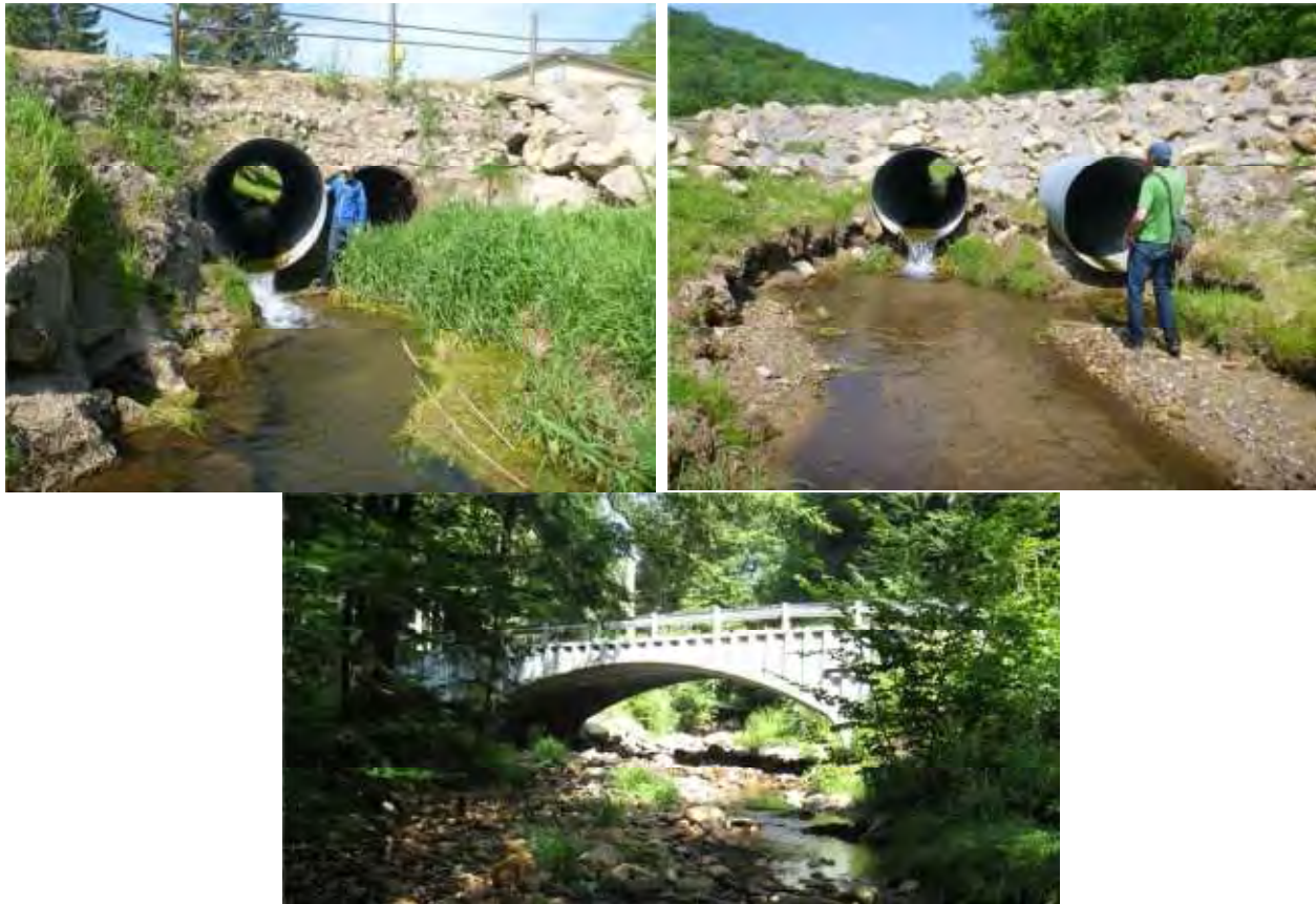
Figure 21. The culverts under both road crossings near the Afton Alps lodge are all perched and undersized, leading to erosion and ecological concerns (top photos). These can be replaced by bottomless arch culverts (left) or bridge spans for better stream flow. (Photos: Inter-Fluve)
