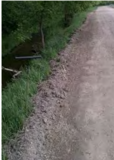
Figure 4. Grading spoil on creek bank (Photo: HR Green)
