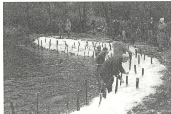
After inserting the willow posts, they can be cut off at 1 to 2 feet above the ground. Erosion control matting is laid down on the reshaped banks to reduce erosion.
