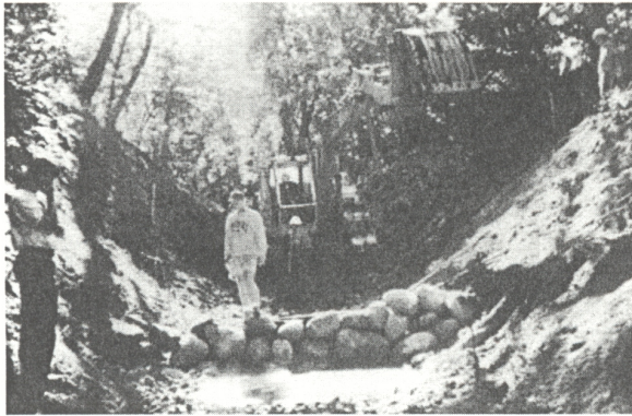
Reducing the gradient in gullies or ravines reduces the erosive force of the water flows. Grade control structures such as this rock weir reduce flow velocities and allow a streambank to reestablish vegetation and stabilize. The rock weir is constructed in the shape of an arc with the high point oriented upstream.
