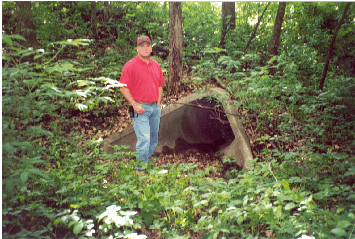
Matt Moore, South Washington Watershed District Administrator, stands by a culvert in subwatershed RL-2, located in the northwest portion of the subwatershed. Not much, if any, runoff from this part of the watershed makes it to Ravine Lake.
